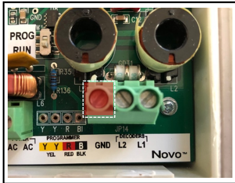
Grounding Terminals for the Novo 2Wire Converter Figure 8-1
