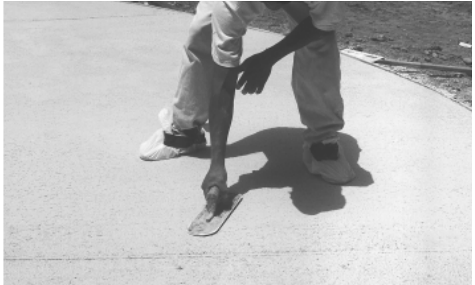
Soft plastic bags allow the finisher to apply the final pass without leaving foot prints.
